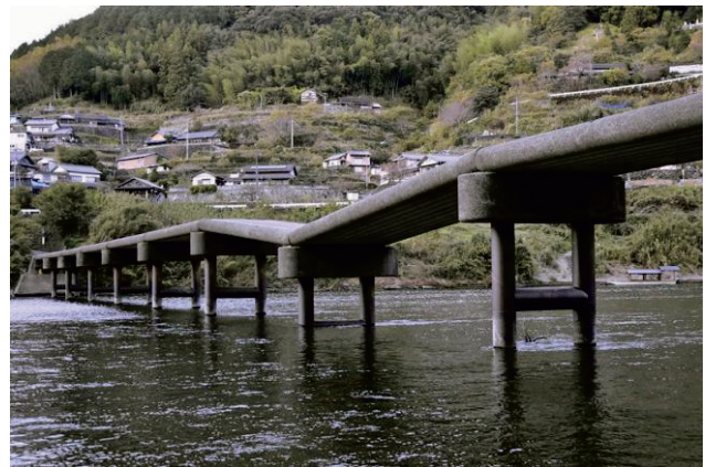
Fig. 2 Collapse of the Iwama Ohashi bridge at its center
