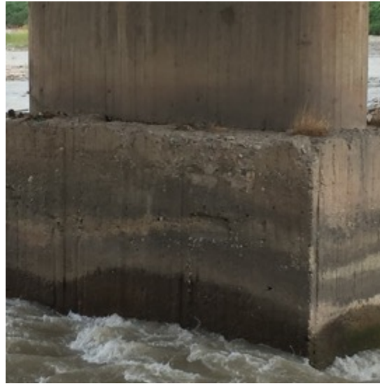
Progression of deterioration
