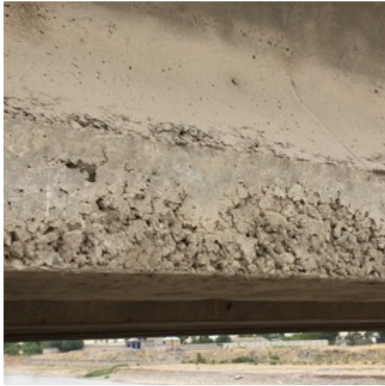
Construction quality issues
