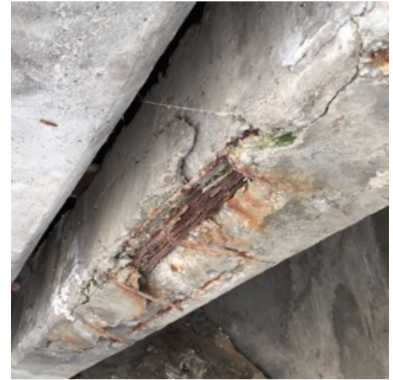
Presence and extent of damage
