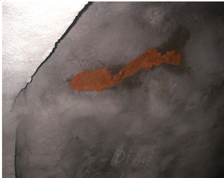
(b) Spalling at Location 3
