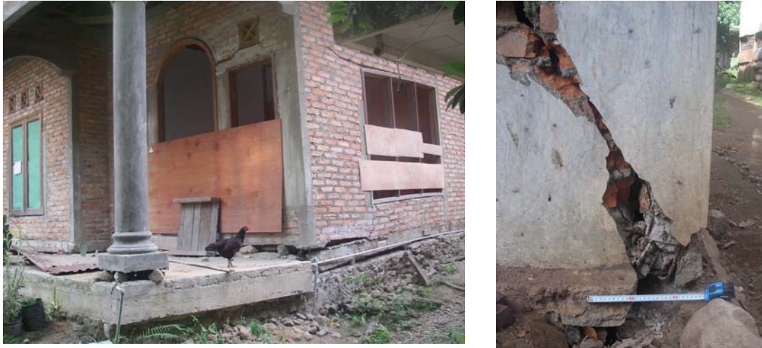
Figure 5.3. Damage induced by surface ruptures to masonry houses with reinforced slabs and columns in Sumpur
