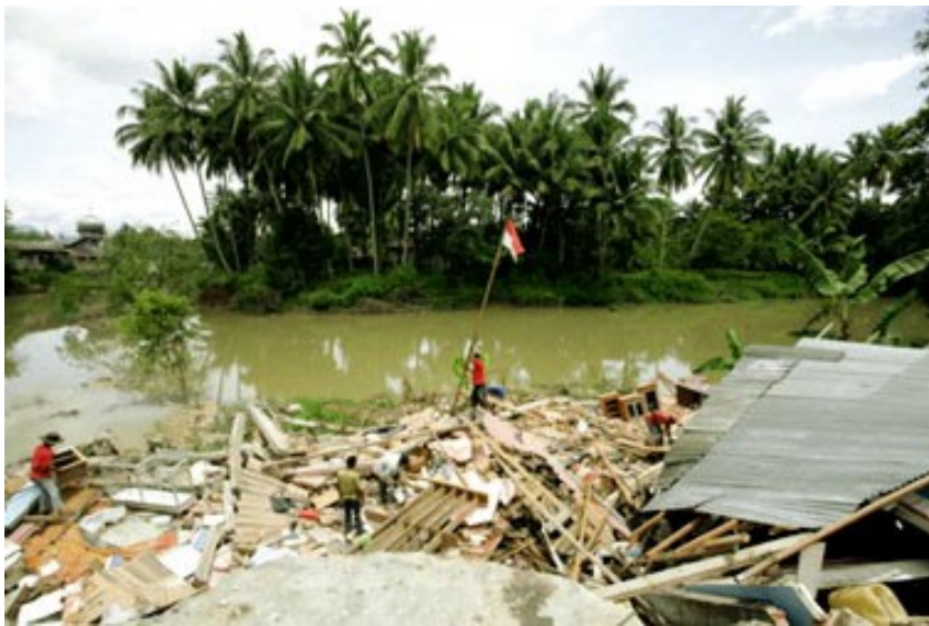
(b) Embankment failure along a river in Solok District Figure 8.7. Some views of embankment failures
