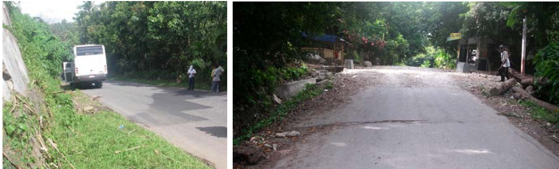
(a) Rupture of roadway in Batipuh (b) rupture of roadway in Sumpur Figure 4.3. Surface ruptures
