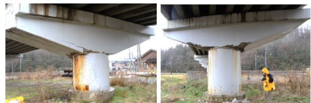
(b) Damage with concrete spalling at the root of the pier overhang
