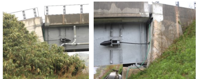
(b) Tilting of bridge abutments
