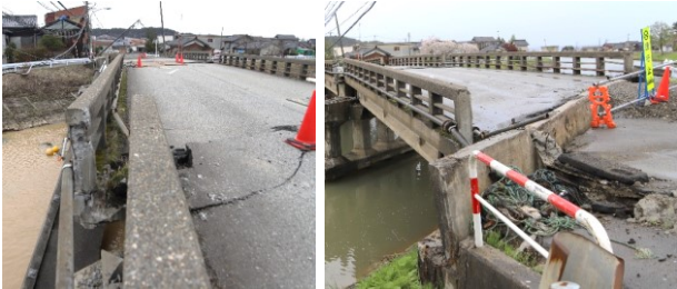
(b) Lateral displacement of vehicular traffic section (c) Step at approaches to bridge
