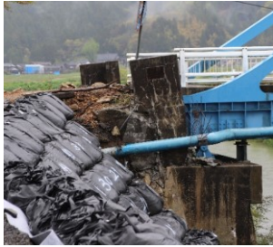
(c) Tilting of bridge abutment
