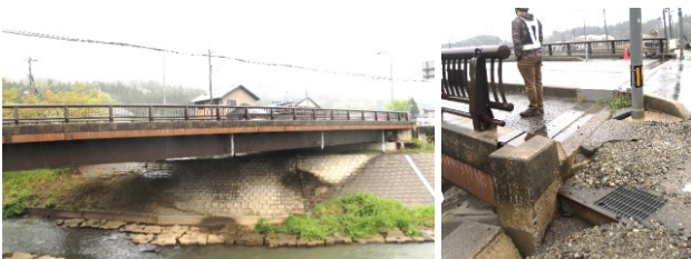
(a) Overall view (b) Step at approaches to bridge
