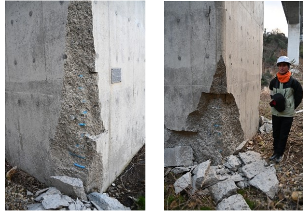
(b) Damage with spalling of concrete and exposure of rebar at the base of pier
