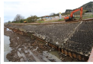
(b) Revetment deformation occurred in vicinity of bridge
