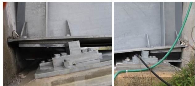
(c) Damage to rubber bearings
