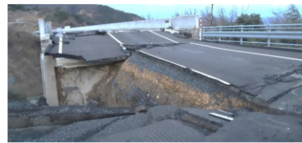
(c) Ground failure behind abutment
