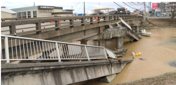
(a) Collapse of the section designated for pedestrian traffic
