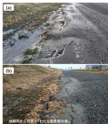
Fig.14(a) Sand ejecta after the 2022 earthquake captured by Mr. aito, a local resident, (b) sand ejecta after the 2021 earthquake at the same location 15)
