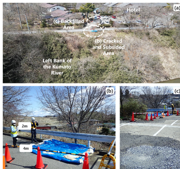
Fig.2 Cracked and subsided area in Yabuki Town of Fukushima Prefecture (a) Whole view, (b) Subsided area of 2m by 4m, (c) Backfilled area in the parking lot
