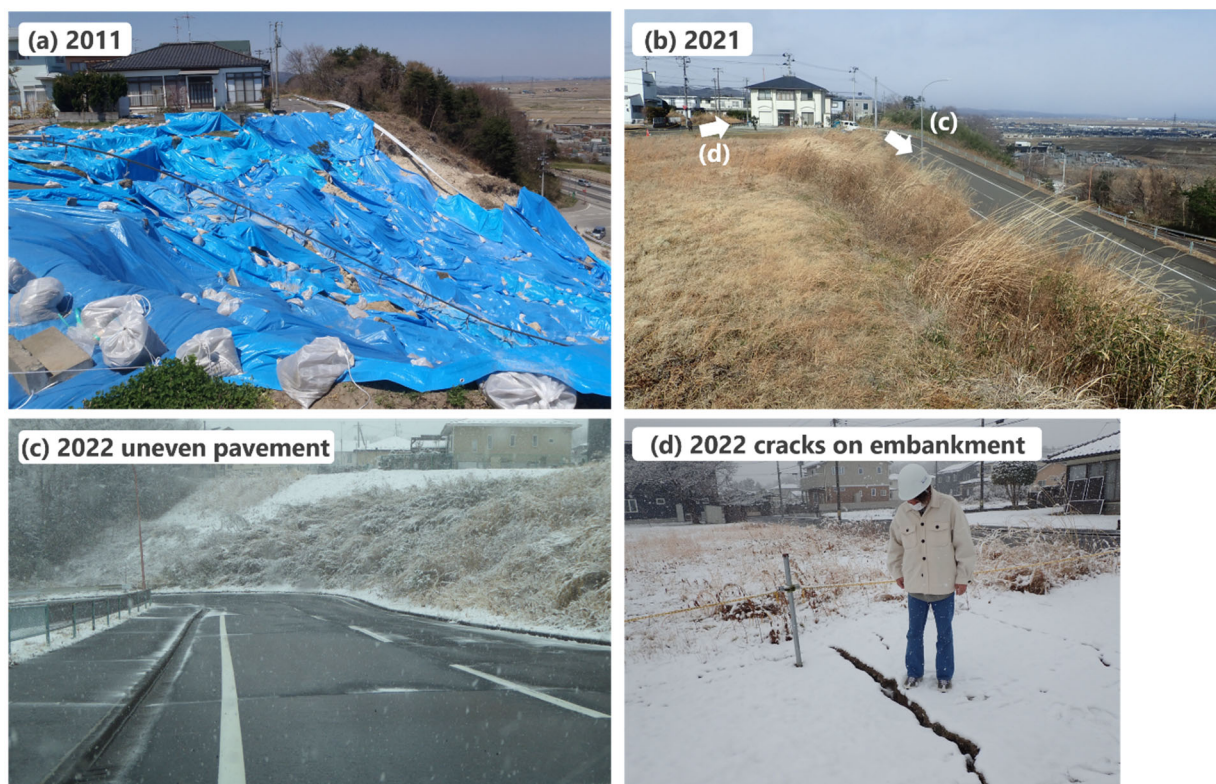
Fig.15 Ground deformation of the slope of Taiyo Newtown (a) after the 2011 earthquake, (b) after the 2022 earthquake, (c) uneven deformation, (d) cracks on the embankment
