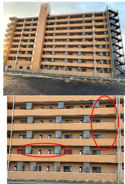
Photo 11 A residential building with SRC structure in Koriyama City. (north elevation, east-west direction)
