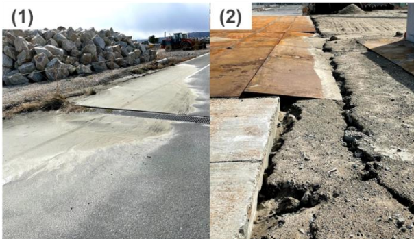
Photo 3 Liquefaction-induced damage in Soma Port
