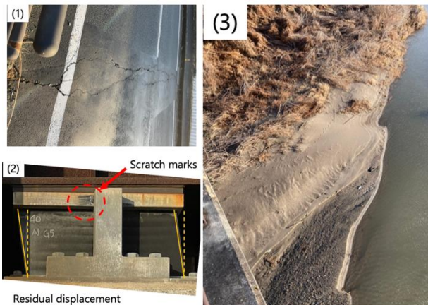
Photo 5 Damage of Soma East Bridge.
