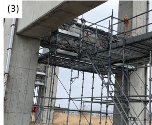
Photo 6 Damage of Shinkansen Viaduct.
