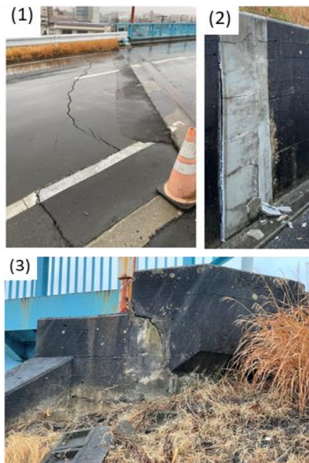
Photo 4 Damage of Soma Overpass Bridge.
