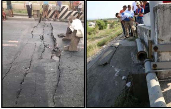
Fig. 8. Damage to Consuela Bridge in Floridablanca, Pampanga (Source: www.bworldonline.com)
