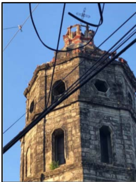
Fig. 14. Damaged bell tower of St. Augustine Church (Source: www.thesummitexpress.com)
