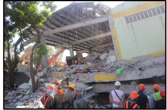
Fig. 10. Observed damages to the Chuzon Supermarket
