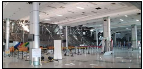
Fig. 11. Damaged ceiling in Clark International Airport
