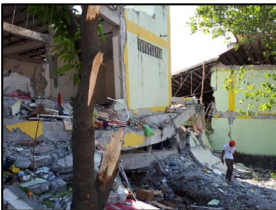
Fig. 9. Damaged exterior of Chuzon Supermarket
