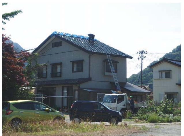
Photo 12 Damage of the tiled roof at Yuatsumi area (N38.615022, E139.60404).
