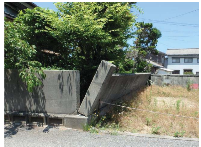
Photo 9 Tiled of the block fence without reinforcement in Fuya area (N38.514325, E139.53343).
