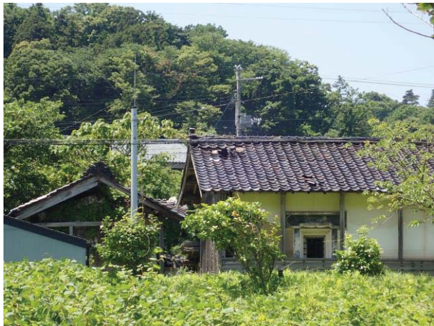
Photo 2 Slightly damage of the roof tile on the wooden house in Kangawa area (N38.451535, E139.496093).
