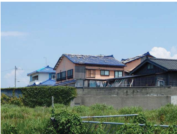
Photo 7 Damage of the tiled roof in Fuya area (N38.516572, E139.533605).
