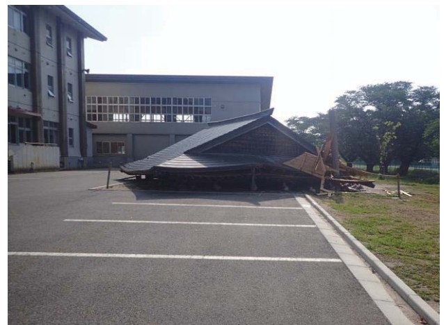
Photo 14 The roof of the Sumo ring in Oizumi Elementary School which collapsed (N38.615, E139.604167).
