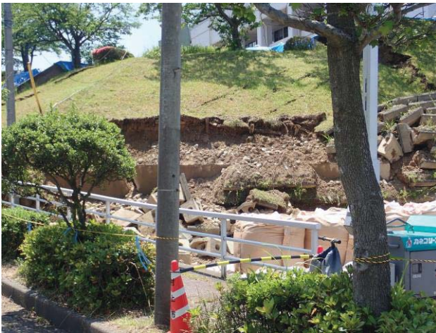
Photo 6 Slope failure of development land in near Fuya station (N38.513557, E139.534312).
