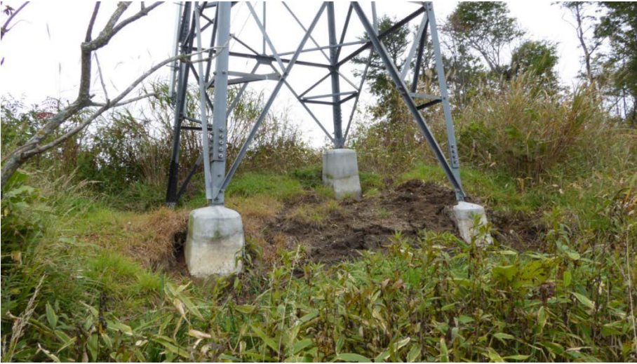
Fig. 6 Slightly exposed foundations of a 66kV transmission line tower (Photo taken at N42.7563, E141.8704 near Point C 3 on Oct. 10, 2018 by Kazuo Konagai)
