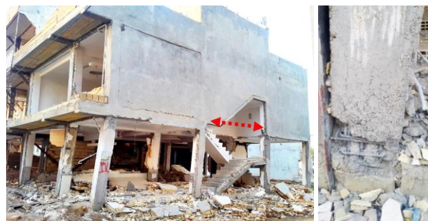
Photo 7 Horizontal irregularities due to lack of one of the beams, poor quality of concrete and utilize of 90° hooks instead of 135° hooks in transverse rebar of columns caused the soft story damage in this building at Sarpole-Zahab.
