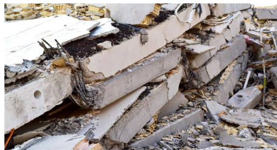
Photo 6 Soft story failure at Sarpole-Zahab city.
