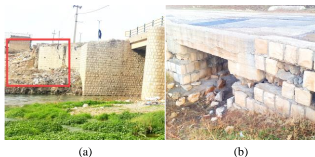
Photo 12 (a) Damage to the retaining walls beside the bridge of Sarpole-Zahab City, (b) Damage to little stone and concrete bridge at a Village road nearby Sarpole-Zahab
