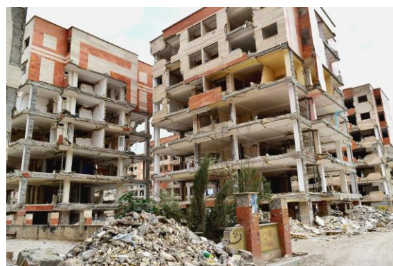
Photo 9 Severe non-structural elements damage at Makane-Mehr of Sarpole-Zahab City.
