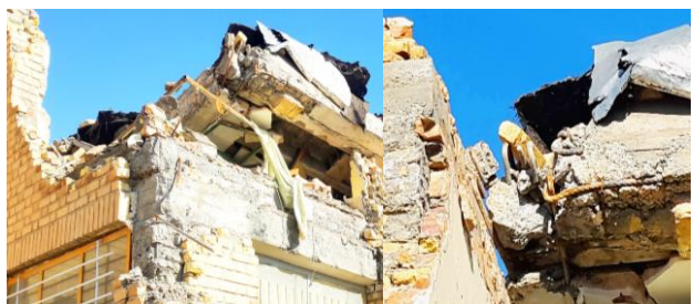
Photo 11 Damage of Esmat Highschool building in Salase Babajani.
