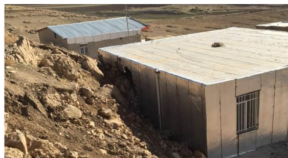
Photo 3 Damaged houses by landslides
