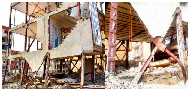
Photo 10 Severe damage to a steel building at Sarpole-Zahab City.
