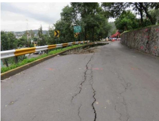
Fig.28 Damage in the Tulyehualco-Xochimilco highway
