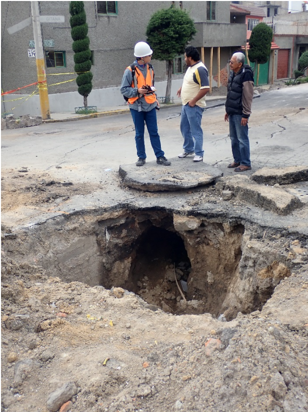
Fig.27 Sinkhole nearby Marist University
