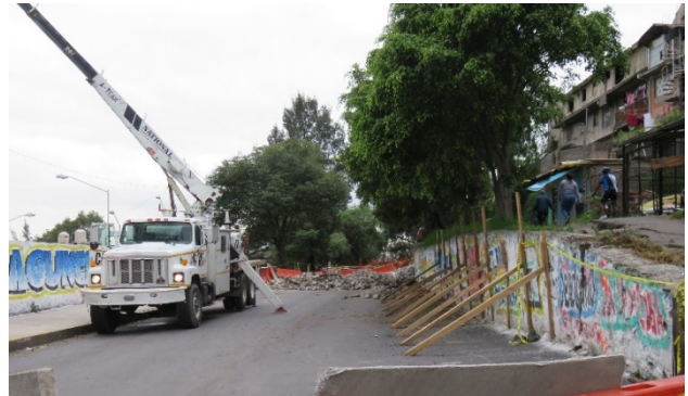
Fig.29 Inclination of retaining walls
