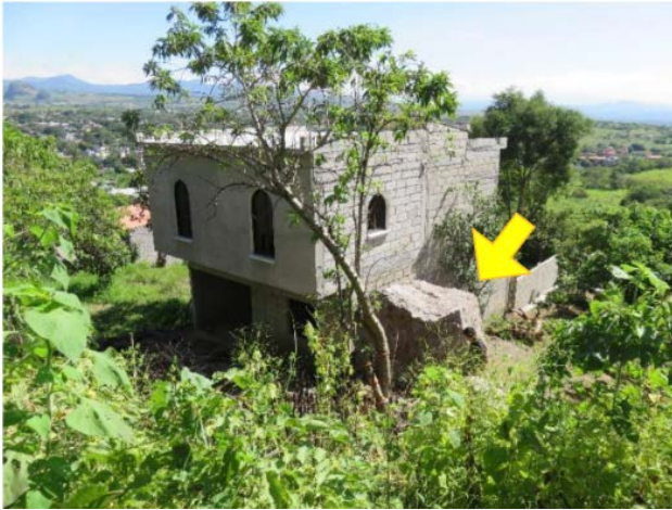
Fig.31 House wall destroyed by rock falling
