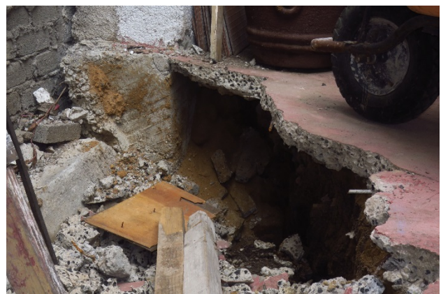
Fig.26 Site 2. Sinkhole inside of the house
